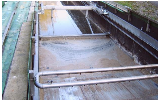
Scum removal with cable pull scraper
